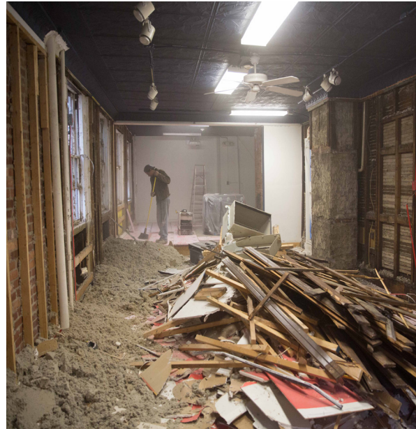
LEFT / Rendering of Social Umbrella concept BELOW / Interior demolition at the EMW Bookstore space
