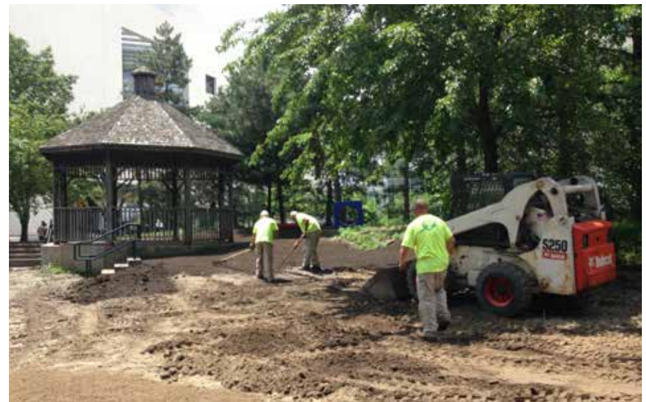
Left: 2013 Budget verses Actual Expenditures Top: The Biogen office building at 17 Cambridge Center was occupied in June. Bottom: Greenscape completes the demolition of the former tot lot at Main Street and Galileo Way.
