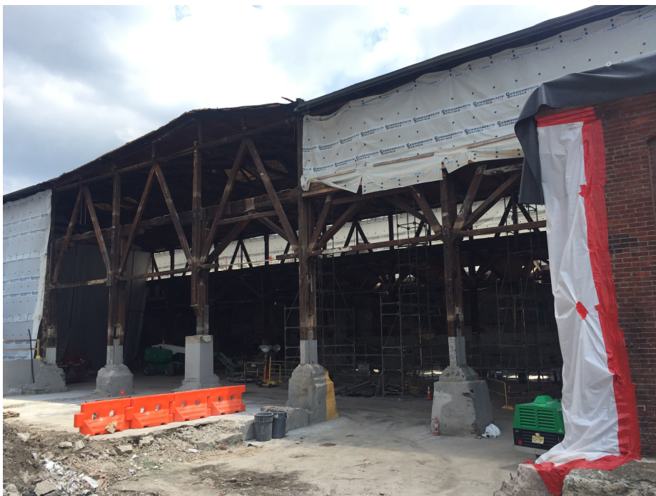
July 9, 2020 view of Foundry from edge of Rogers Street, by Verizon property. The structurally unsound addition has been removed.
