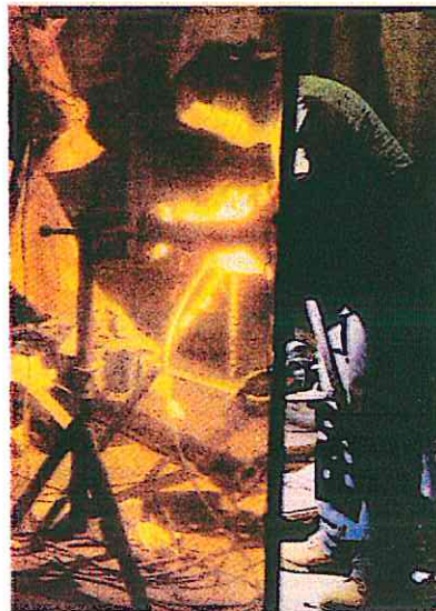
Welder works on installing BiogenIdec's power plant in a building in Kendall Square
