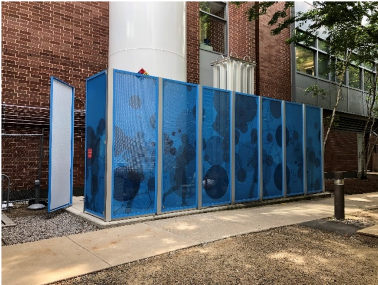
Tank Enclosure at Biogen Building 6, 115 Broadway, Cambridge
