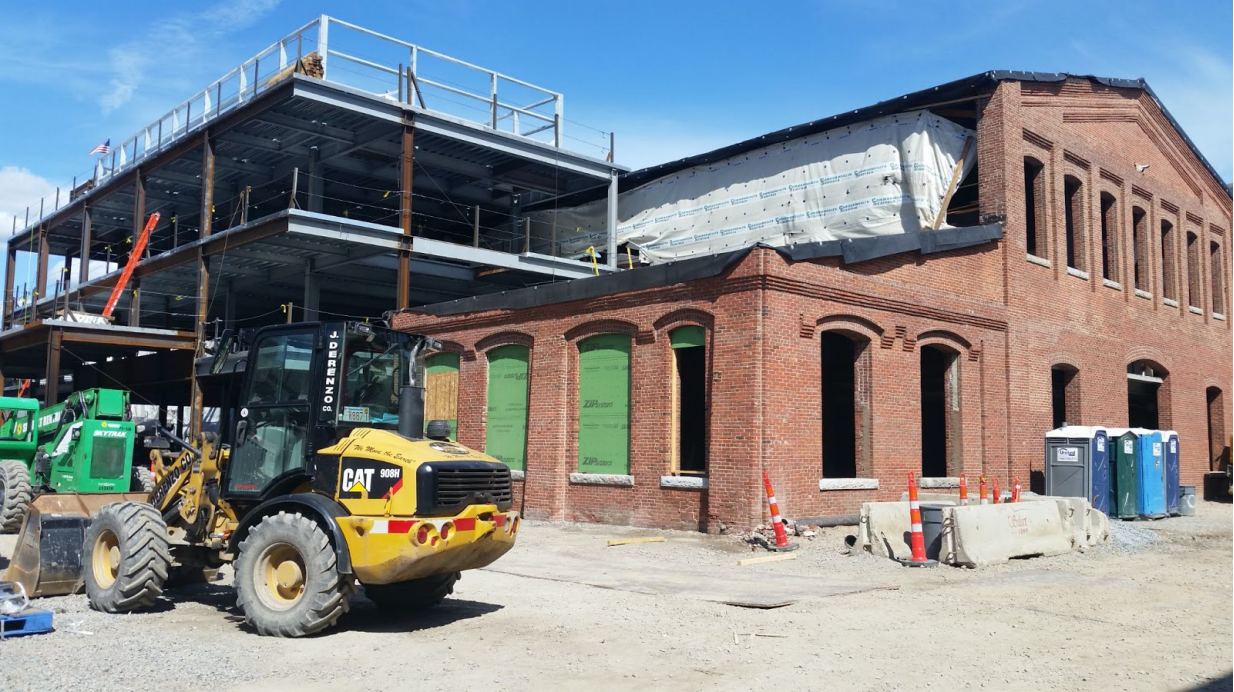
Foundry - Foundry construction remains on time to be substantially complete by May 31, 2022, with all punch list items completed by July 31, 2022.
