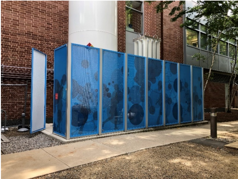
Tank Enclosure at Biogen Building 6, 115 Broadway, Cambridge
